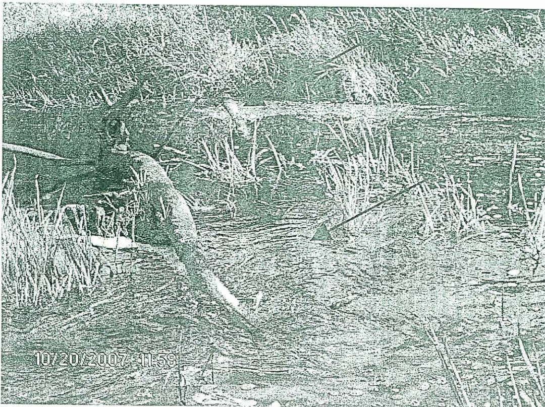
View of pipe spanning river about 10 yards downstream from Chip Rd. bridge, looking east.
